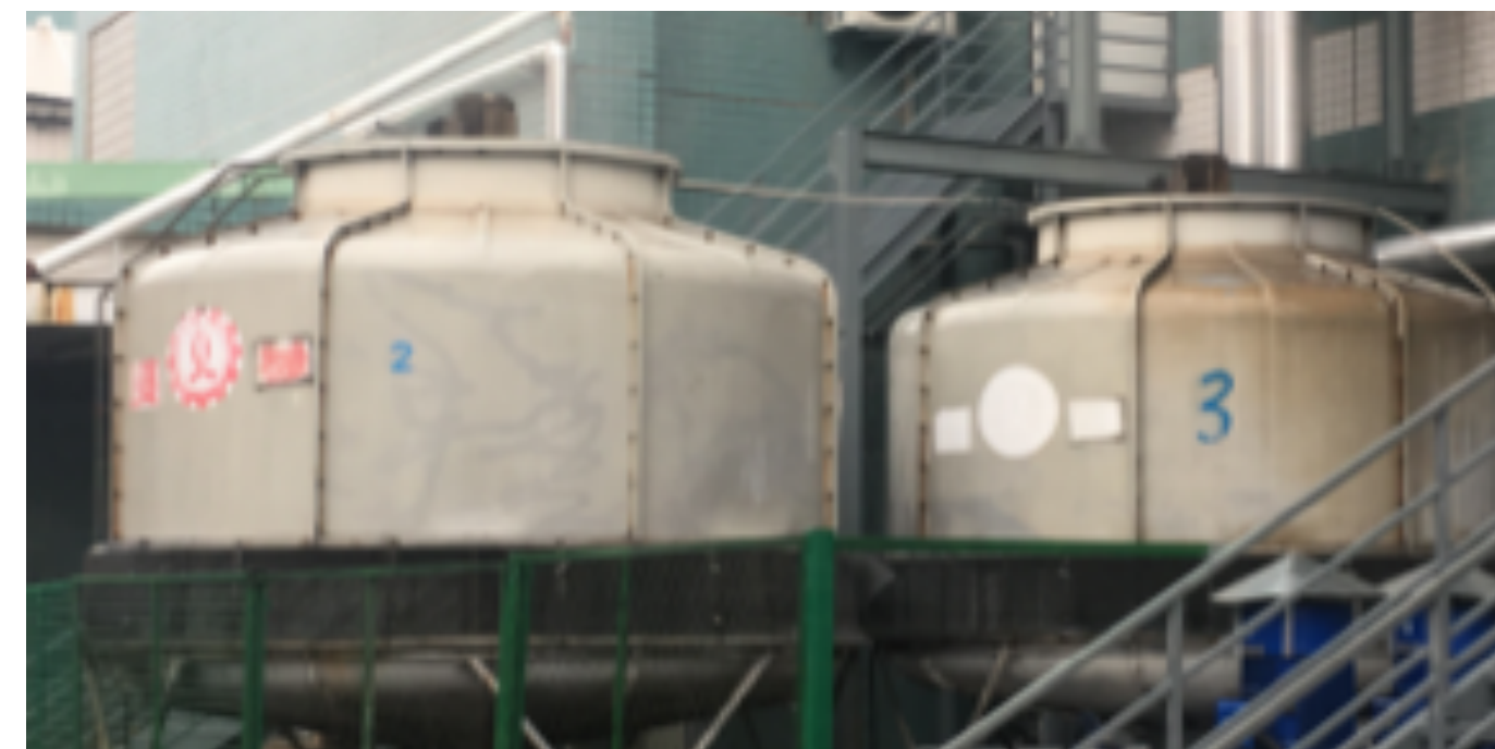
Figure : Cooling system for processing recycled water
