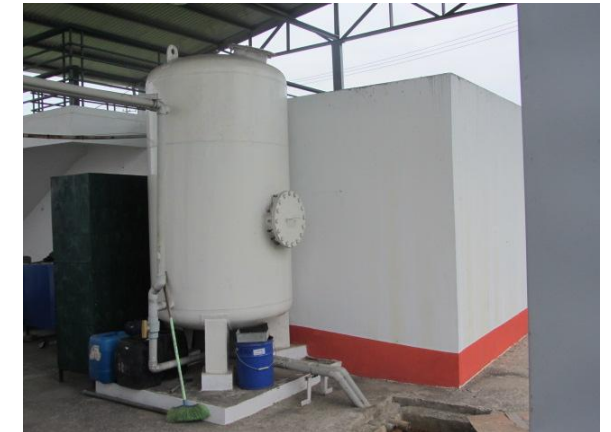
MPT Vietnam filtration water tower
